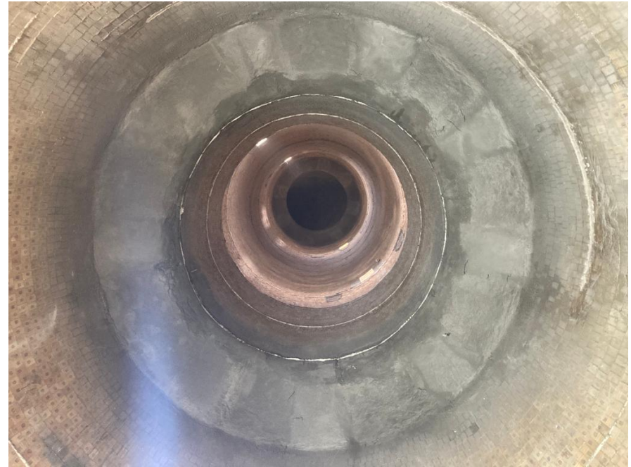
Refractory inside New Calciner
